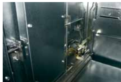
Interlock for circuit breaker compartment door
